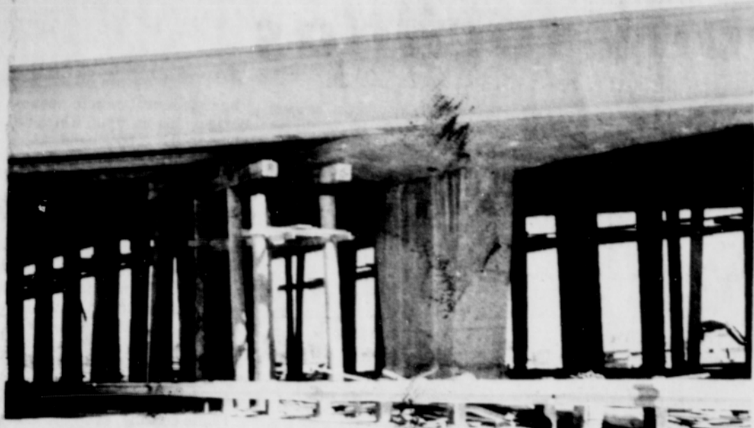
WORK IS again progressing on the Boring Rd. interchange, "Blood Alley". The work was started over a year ago, and most recently has been delayed by a construction strike. The intersection got its name "Blood Alley" following several deaths caused by accidents. (Post photo)
