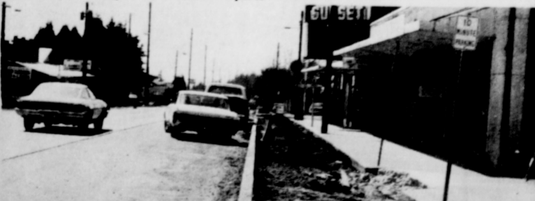
THE CURB work along the north side of Proctor Ave. was the first part of the improvement project. The crews are now working on the south side curbs. Once the
