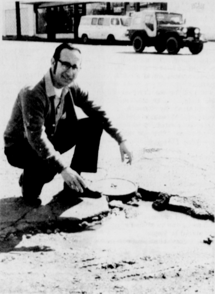
JOE ASTLEFORD, Street Commissioner on the city council, points out a particularly bad pot hole near Proctor Avenue. This and others will be repaired when Proctor is redesigned and improved this spring. (Post Photo)
