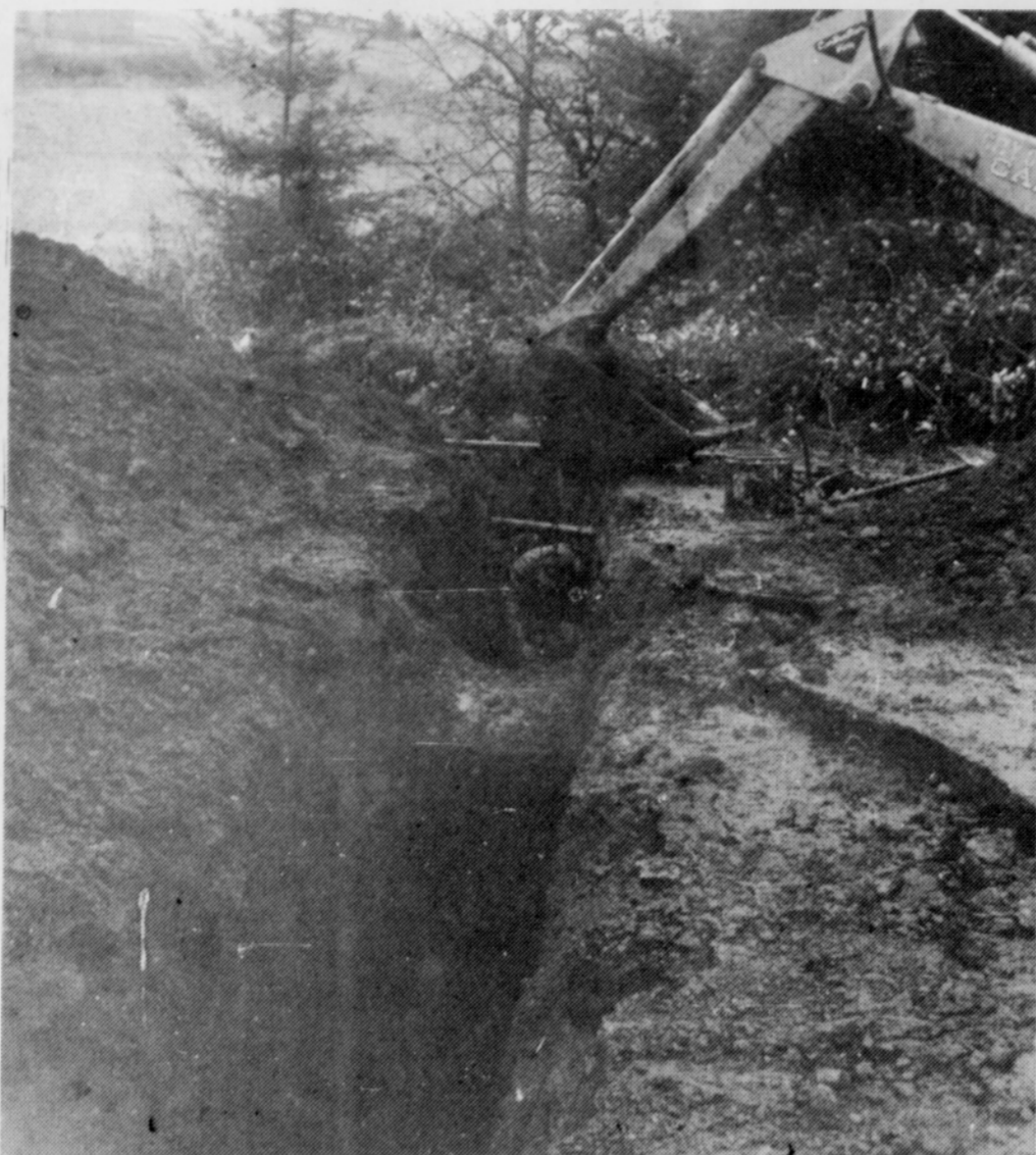
THE SANDY city crew has been busy during the past week installing the sewer line to the apartments on Third St. which were recently completed. The street has
