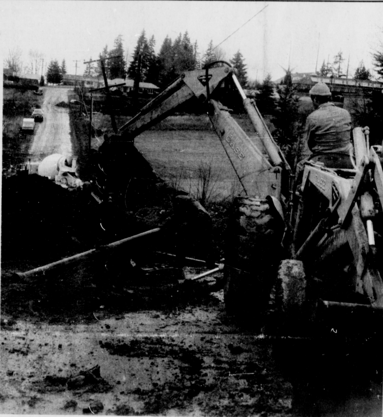
THIRD AVE. in Sandy has been blocked off down to one lane of travel during the past week as city crews complete installation of the sewer line to new apartments on the corner of Pleasant St. and Third Ave. Here
