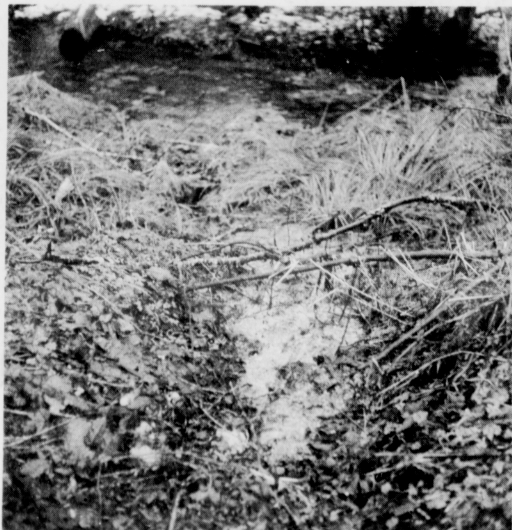
ACCORDING TO county officials the Rhododendron area is the first area which must have sewers in the mountain area due to its high sewerage runoff already. Sewerage from a septic tank can be seen draining into Little Brook. A petition is
