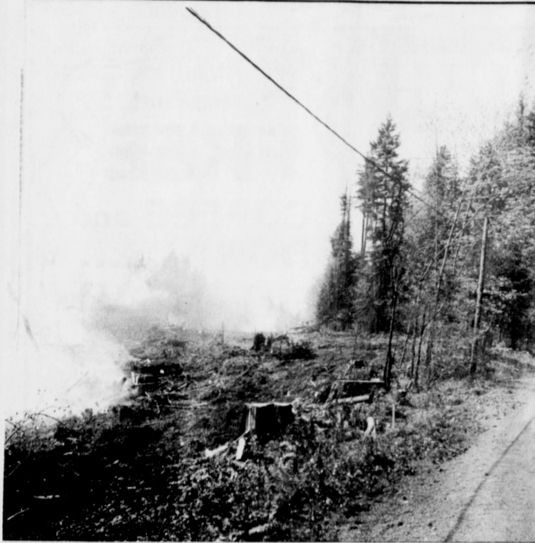
EVIDENCE OF PROGRESS for the Hoodland area, is the new four-laned highway which is now under construction between Aldercreek and Wildwood. The above picture was taken near Wildwood. (Post Photo)
