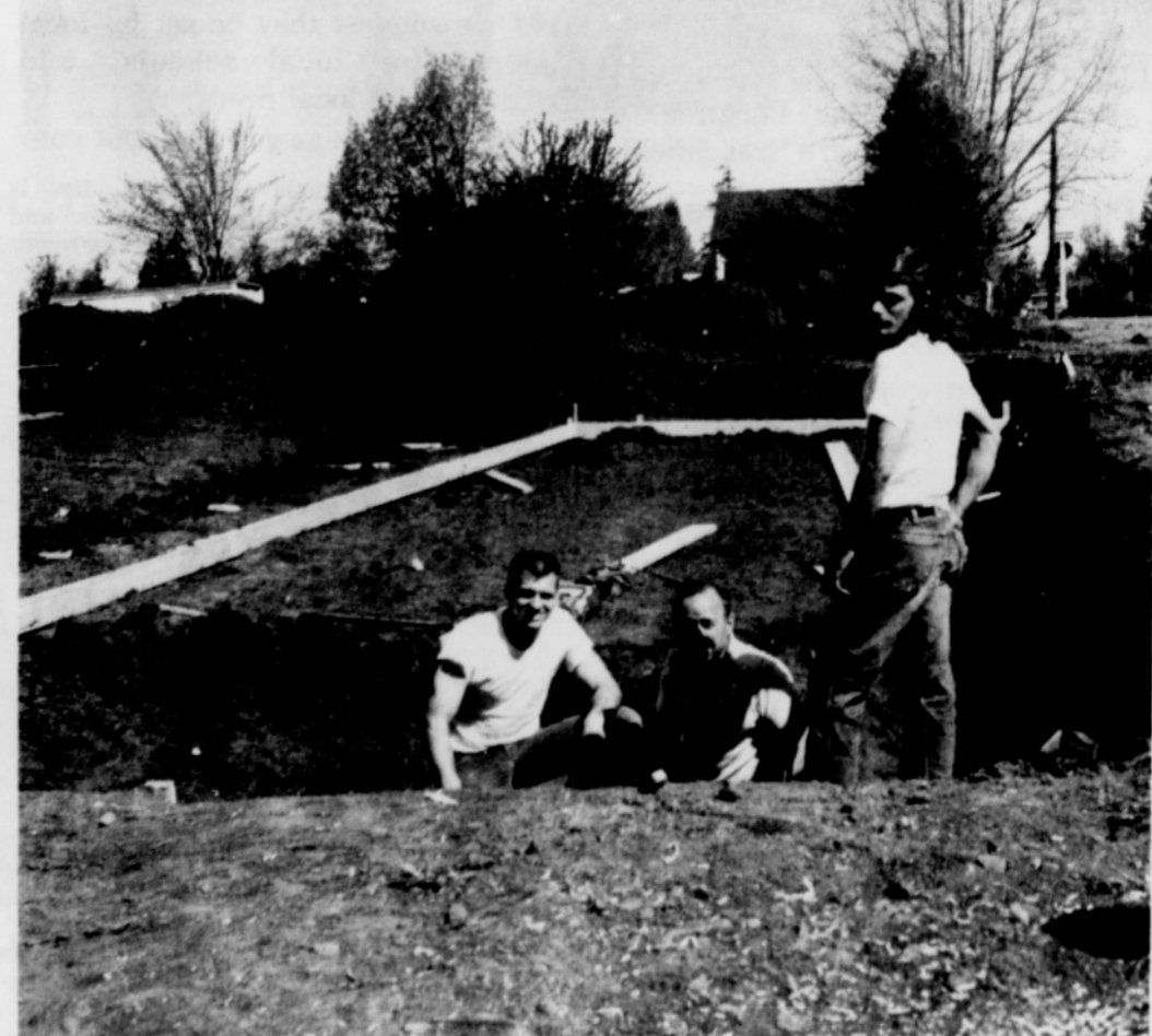
CARL LEATHERS, center, owner of the Leathers Oil Company, broke ground for a 12 pump station Monday. It will be located between Center, Main and Proctor Streets, and will extend behind the Big Apple Store.
