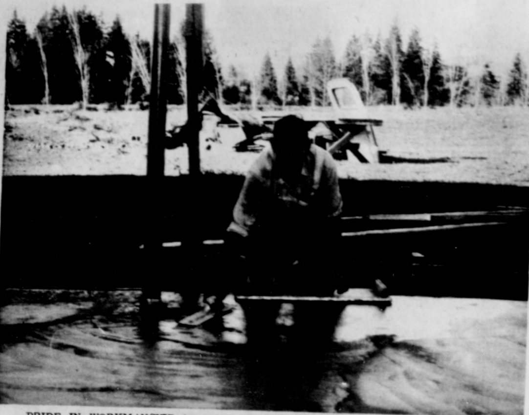
PRIDE IN WORKMANSHIP is not dead, and here Merle Tolson smoothes the newly poured concrete slab at Janz Fruitland, now Plantland. Bob Pullen and Denny Grey along with Mr. Tolson have taken advantage of the fine weather to build additional display space for their expanding business.
