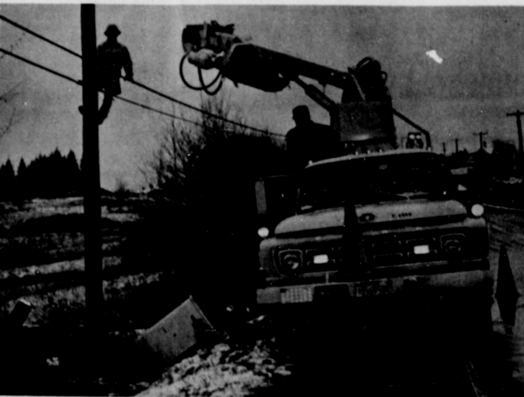
A telephone pole about two-tenths of mile west of Mt. View Lumber Company on Loop Highway 26 was snapped in two sometime Monday night by a motorist. Crewmen from West Coast Telephone Company have replaced the snapped pole with a new one here and preparing to hook telephone lines to it.
