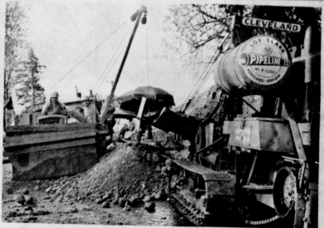
Digging a trench, laying sections of pipe line and covering it was moving along at the rate of 13 to 18 feet per minute last week in this area located about 1.7 miles from Boring. When completed, about the middle of November, residents of the area will be able to use natural gas heating here for the first time. (Post Photo)
