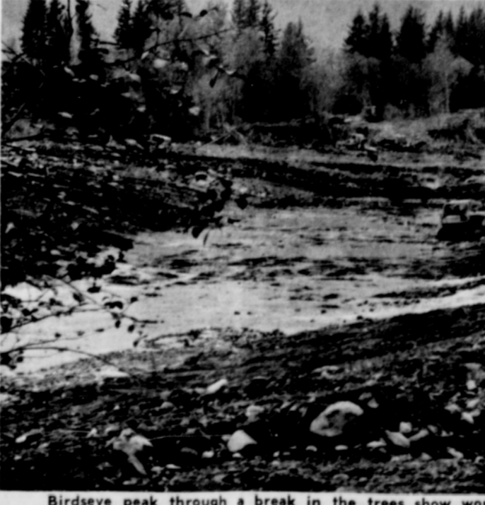
Birdseye peak through a break in the trees show work on the original channel of the Sandy River near Wildcat Creek. As many as 14 D-8 cats have been counted at one time working in this area. Following work by the cats waters will be brought back into the channel as it was before the floods. (Post Photo)
