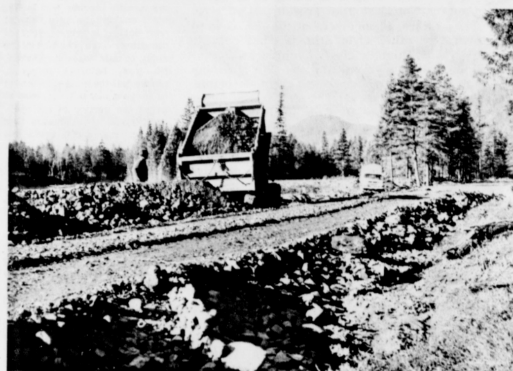
Tons of base rock has been hauled into this county road, Larson Road, by dump trucks as restoration of county and private roadways continue in the damaged Hoodland area. Most county roadways have been restored to at least temporary traveling at this time. Work crews have worked long hours and six days a week to provide access routes in and out by local residents. (Post photo)
