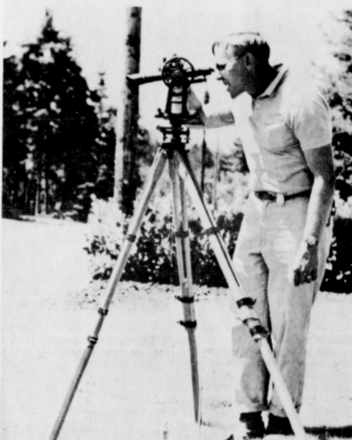
With the relocation this week of the PGE poles, work will soon begin on the surfacing of First and Scenic Sts. Above, Don Boatwright completes surveying for curbing on Scenic. (Post photo)
