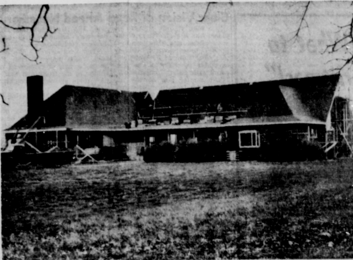
A new religious education center takes shape on the campus of the Women's Christian Temperance Union Children's Farm Home near Corvallis. It replaced the chapel leveled by flames last July. Howard Berger of Sandy is a director of the home.
