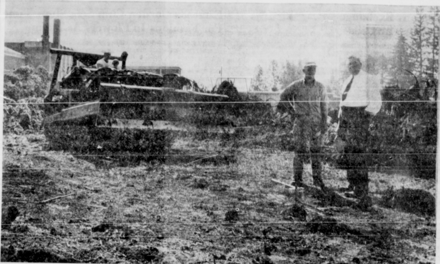
SANDY—Corkum Construction company started building the new Sandy grade school unit here last week. The building is expected to be finished by December. There will be room for three class rooms in the building in addition to a boiler room
