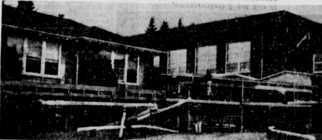
Workmen in the above photo are shown putting finishing touches to the covered walkway between the two Sandy High School buildings. The structure, built at a cost of $3,500, was completed at the end of last week. It is to be painted white when weather conditions permit. Carpenters who worked on the covered walk were S. M. Currie, John Dunn, E. P. Smith and J. A. McReynolds. It was started about three weeks ago.
