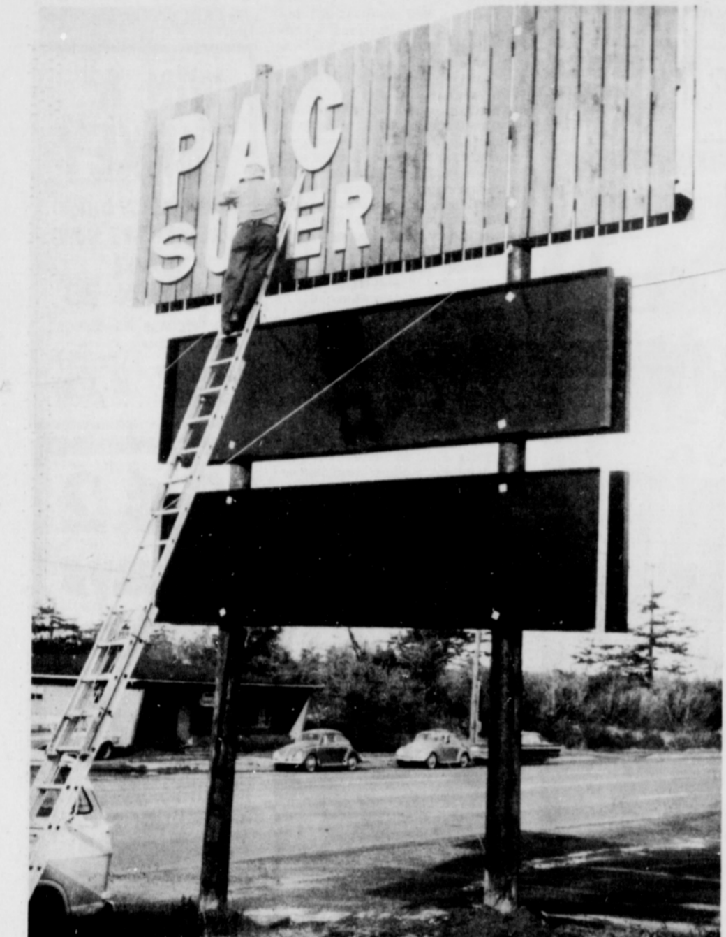
PROBABLY the largest sign in the city went up last week at Pacific Super Market. The sign is designed to carry current specials at the store, besides the store name. In addition, said store owner Jim Peterson, we will use the sign as a community bulletin board as much as is possible. The message now carried announces the coming Christmas Bazaar set for December 3.
