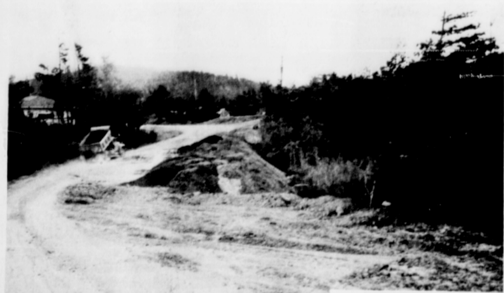
NEW FILL is going in on Lakeshore Drive to fill in swamp area and widen road. Fill dirt is coming from the south end of Oregon St., being opened to standard city street width and cut to grade.
