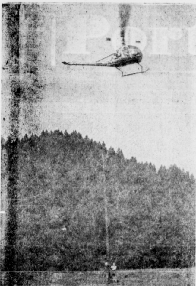
Ground crew appreciates the services of helicopter as they construct power lines to serve the Agness area. Collins Electric of Salem are the contractors, and are building the line for Coos-Curry Electric, thru some of the roughest terrain in the state. Power in Agness is expected very shortly.
