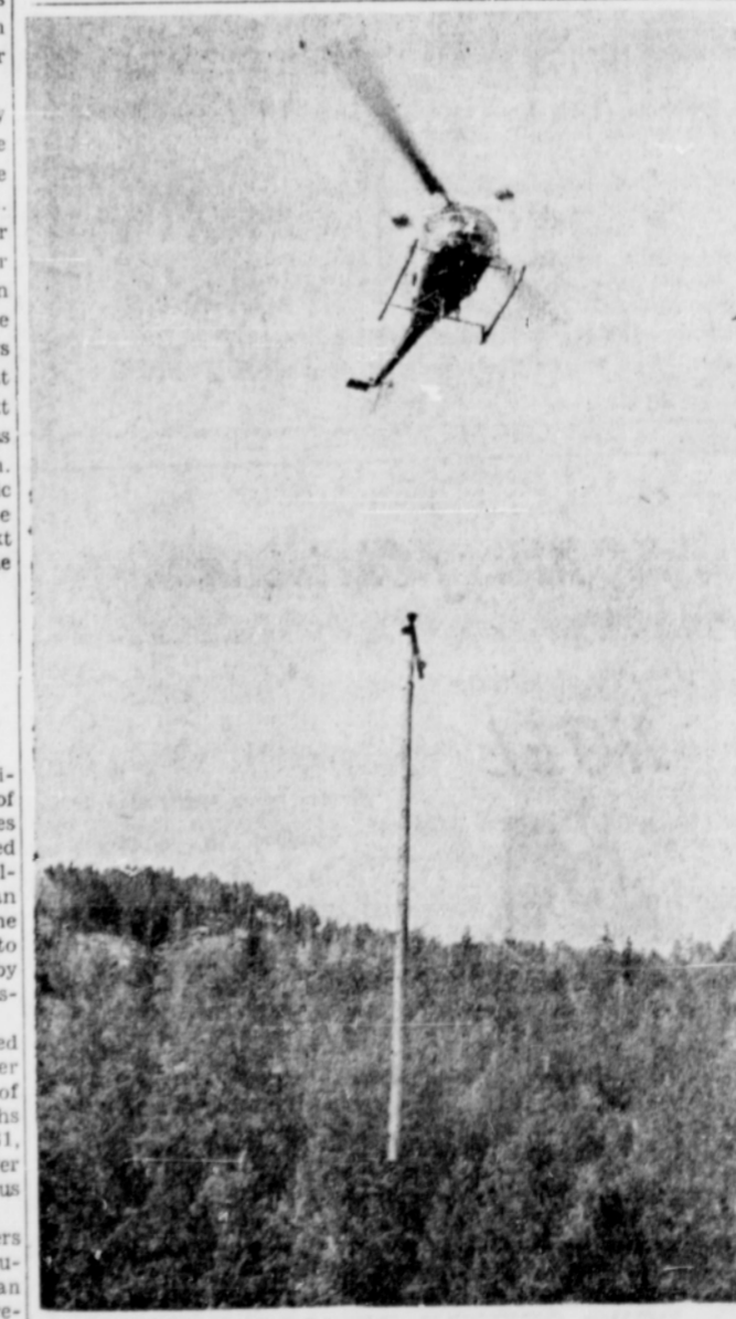
This helicopter proves invaluable in setting poles and stringing wire in rough terrain, as Coos-Curry Electric power moves on to Agness, Collins Electric is constructing the new line.
