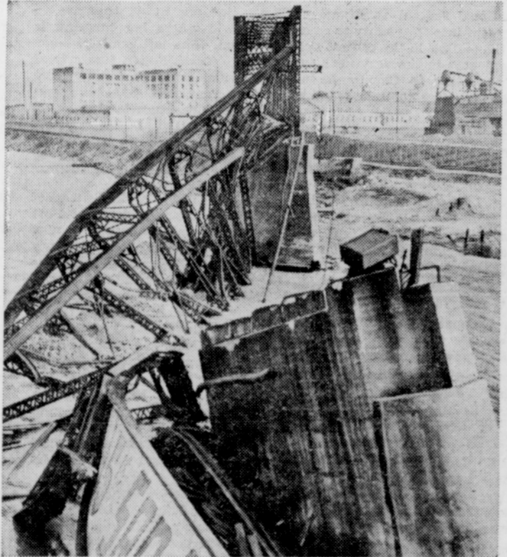
Lashing torrential rains have made this Los Angeles' wettest season in 48 years. The floods undermined and ripped off half of the Santa Fe railroad bridge (shown above) across the Los Angeles river, closing streets and highways with landslides. Hundreds of automobiles were stalled in floodwater.
