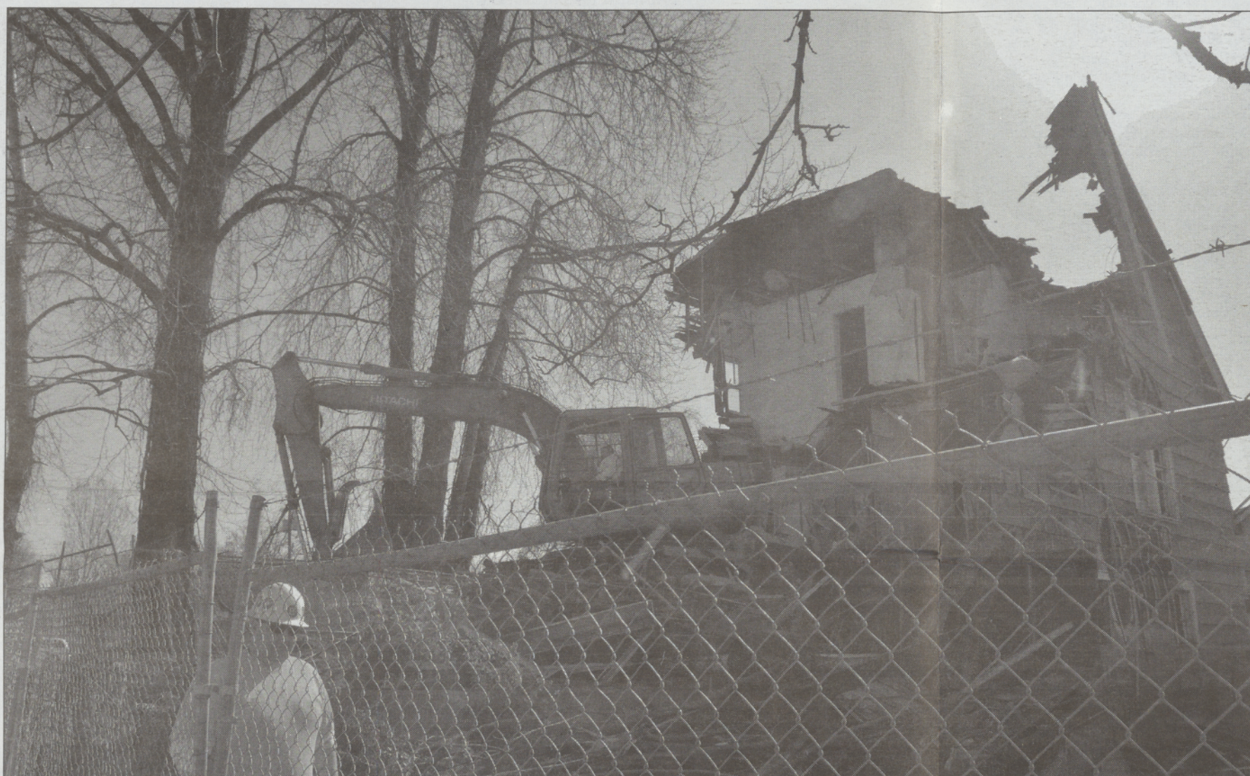
A home is demolished in Northeast Portland, part of a gentrification trend that began in the 1990s.
