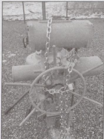
After closing the valve, Higgins chained and locked it in the off position.
