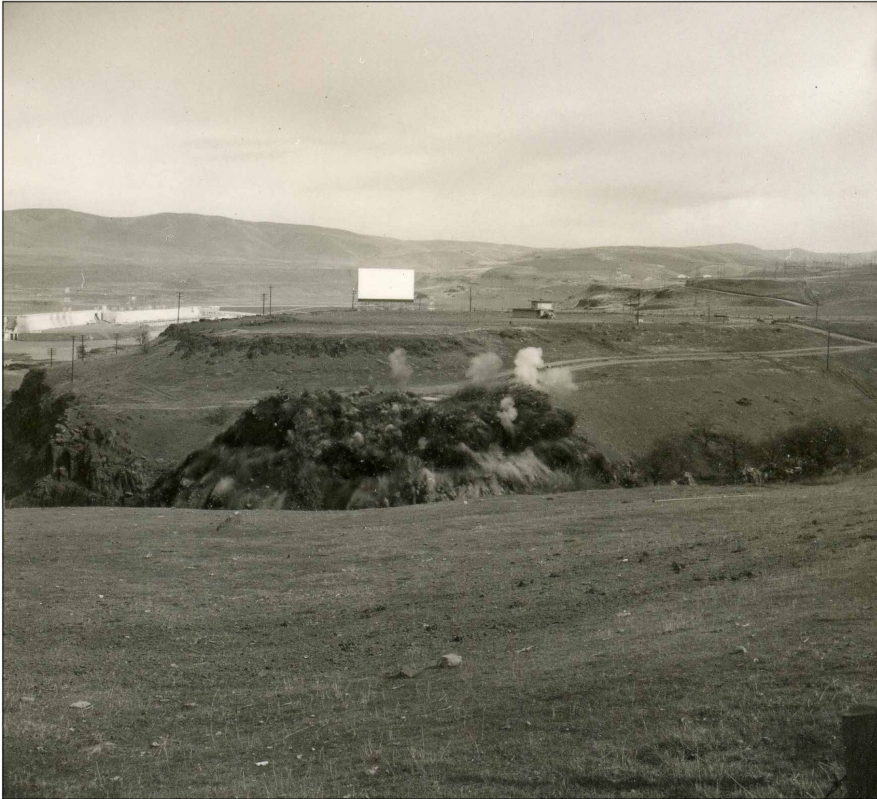
A blast is triggered during work to relocate Highway 197 in The Dalles March 2, 1959.
