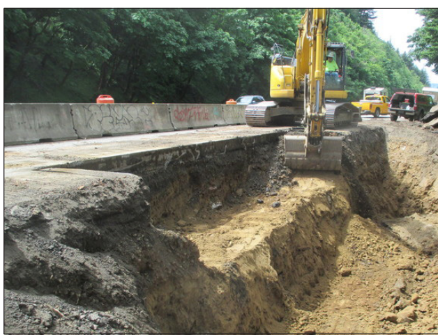
Crews excavate a section off the shoulder of I-84 west and created bench cuts along the slope. These bench cuts, which resemble stairs, are filled with rock to help secure the embankment and the highway shoulder.
