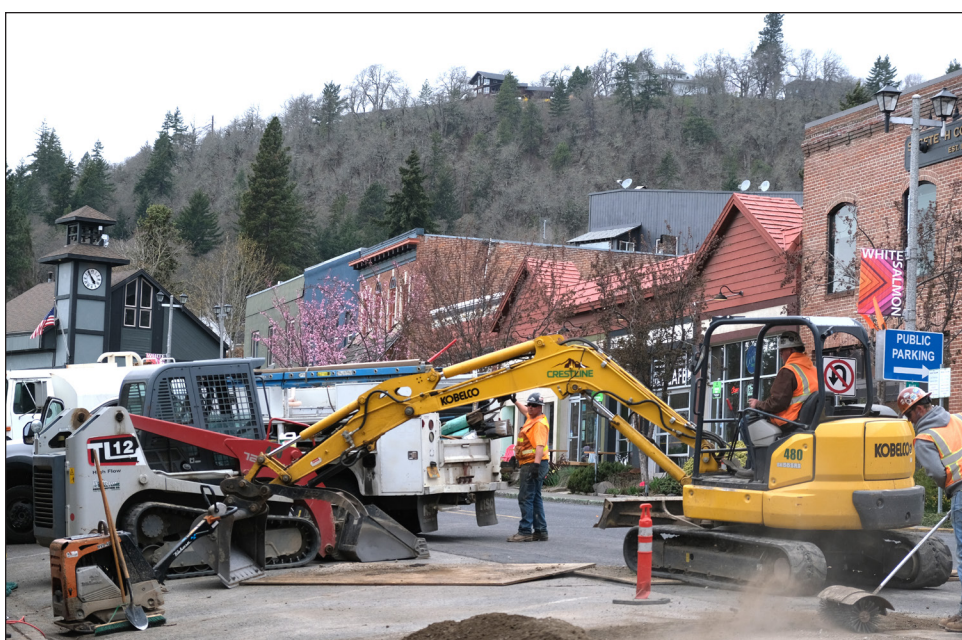
Crestline Construction crews work in early 2020 to replace water main lines in the downtown core of White Salmon. The City of White Salmon recently approved closing the project, and secured a USDA loan that funded the project with a $2.73 million water revenue bond.
