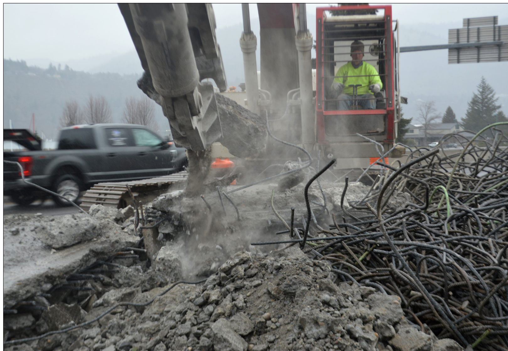
Carter and Company “muncher” machine, resembling a giant metal horse head, pulverizes 12-foot pieces of bridge deck that crews cut up with saws and torches.
