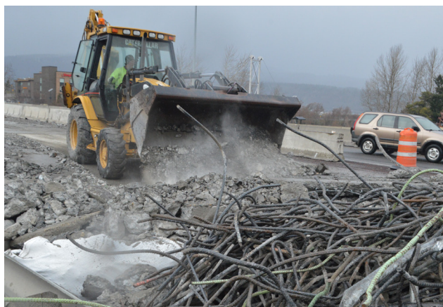
Above left, a load of debris is piled up after the “muncher” machine pulverized the concrete and separated the rebar and other metal. Above right, Steel beams are exposed and an auger perforates another concrete section of Interstate 84 near exit 63 in this view looking east in Hood River.
