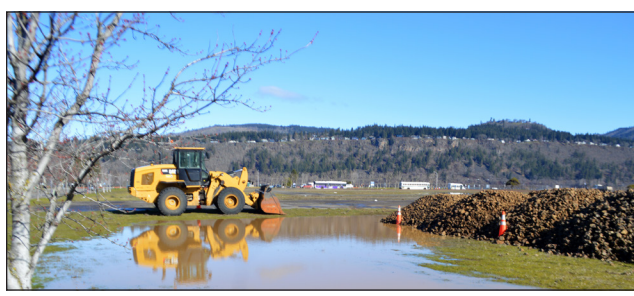
Rock piles are forming at Lot 1 in Hood River, one way the port is helping haulers offset potential increased costs of using the Hood River-White Salmon Bridge.
