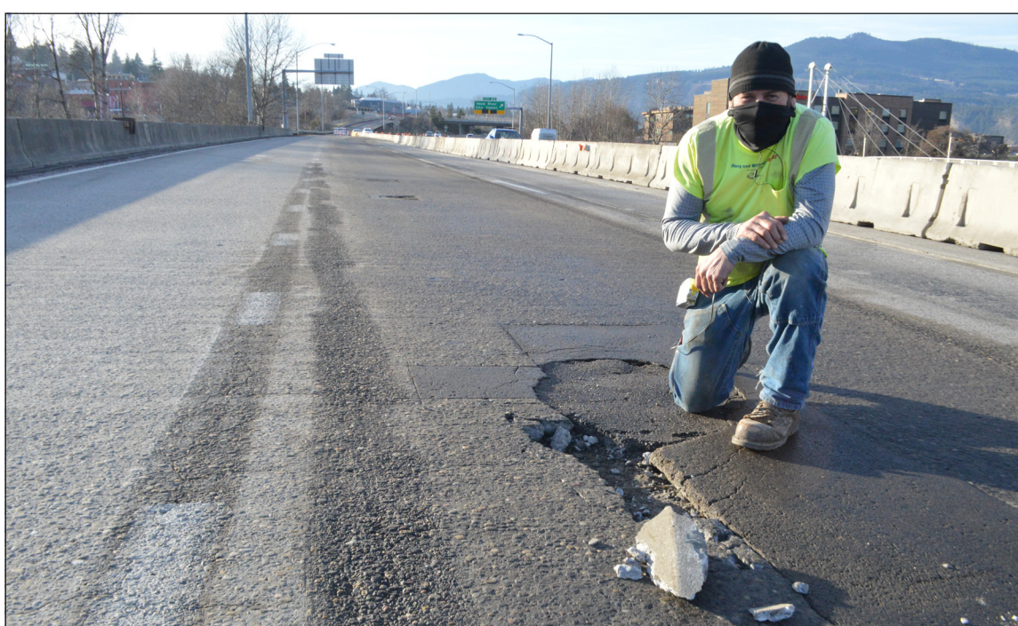
Supervisor Jim Califf with the largest of the holes on the Interstate 84 bridge deck, about 100 yards east of exit 63. Kirby Neumann-Rea photos
