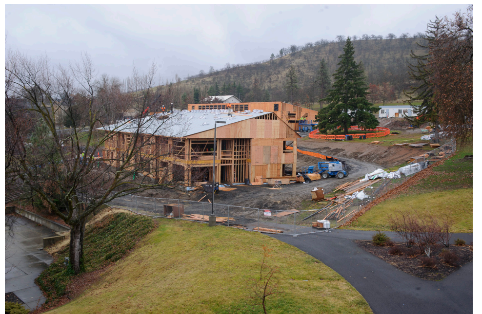
Work on a new residential hall, in foreground above and at top, is well underway at Columbia Gorge Community College The Dalles campus. The workforce skills center, in background above, is also on track. Both are scheduled to open for Fall term 2021. Flora Gibson photos
