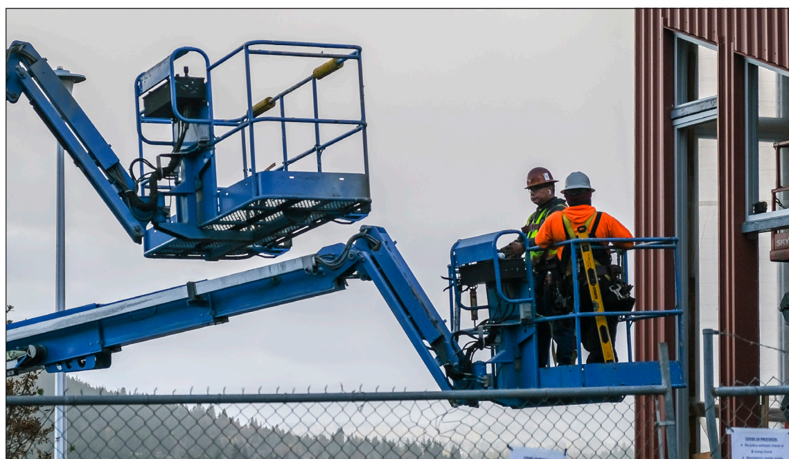
Construction workers were putting up drywall Wednesday afternoon. According to superintendent Christopher Douglass of construction firm Howard S. Wright, work on the roof is substantially complete, and phase one of the project is set to be complete in January. Jacob Bertram photo
