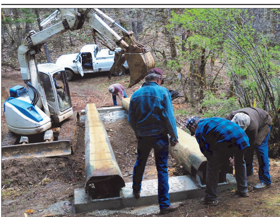
Community volunteers were working early this week through Wednesday, April 21 to construct a bridge at Illinois River Forks State Park, on the south side of Cave Junction. As part of the effort, backers obtained 35-foot long logs. (Photo provided)
