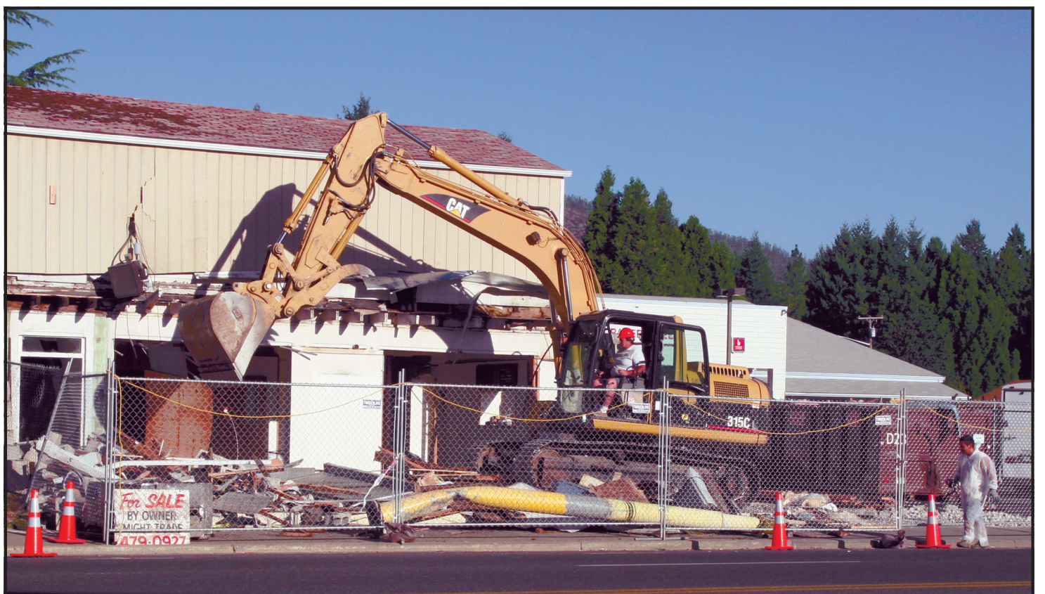
PARTIAL DEMOLITION is under way preparatory to rebuilding the portion of Pizza Pit pulverized July 1 when a motorhome towing a car crashed into it. Work
