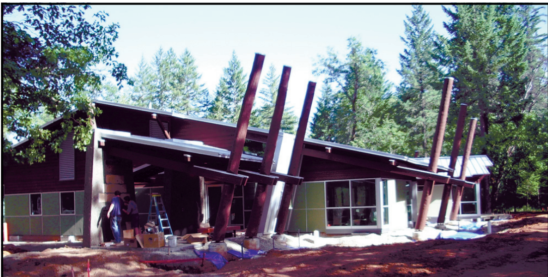
A NEW MEDICAL FACILITY being built at the north end of the city of Cave Junction as the new home for Siskiyou Community Health Center is to open this coming fall. Part of the building will offer services including X-rays by Three Rivers Community Hospital. A benefit for construction costs, Savor the Valley, will be held Saturday, June 24 from 4 to 8 p.m. at Bridgeview Vineyards Winery on Holland Loop in rural CJ. The ad is on page 16. (Photo by 'Illinois Valley News')
