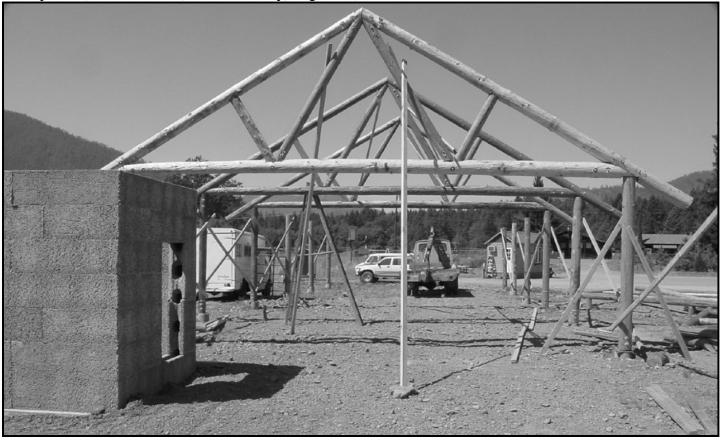
WORK IS PROCEEDING on a pavilion for the Selma Farmers Market at Selma Community Center, the former Selma Elementary School. The market, with fresh
