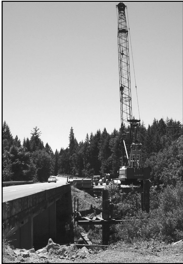
BRIDGE WORK - Three new bridges over the Illinois River and its forks are being built in Illinois Valley by Oregon Dept. of Transportation. The $15 million project includes the work shown above on the south side of O'Brien. ( Photo by 'Illinois Valley News')
