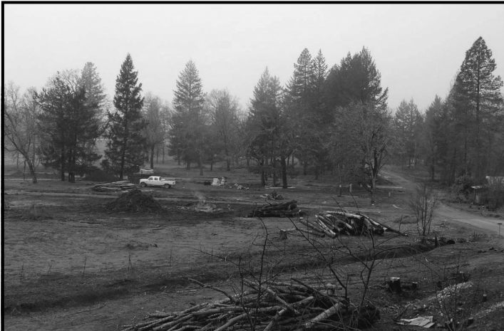
There's lots of residential construction activity in the city of Cave Junction. (Clockwise from bottom left) Daisy Hill Road work, Echo Park on Schumacher
