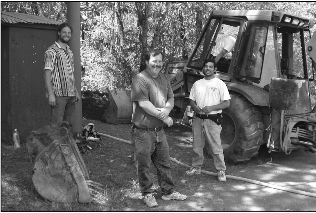
SHINING STAR POWER - (From left) Shining Stars board member Arley Tree, Josephine County Parks operations head Steve Schalk, and JoCo Parks employee Tony Ruiz take a break from their work digging trenches and running conduit for a new 200-amp power service in the Mallard Loop area at Lake Selmac. The Shining Stars, Iron Horse Rodeo, Kerby Electric and PP&L donated money, resources and labor to complete the project before summer festivities. (Photo by Michelle Binker)
