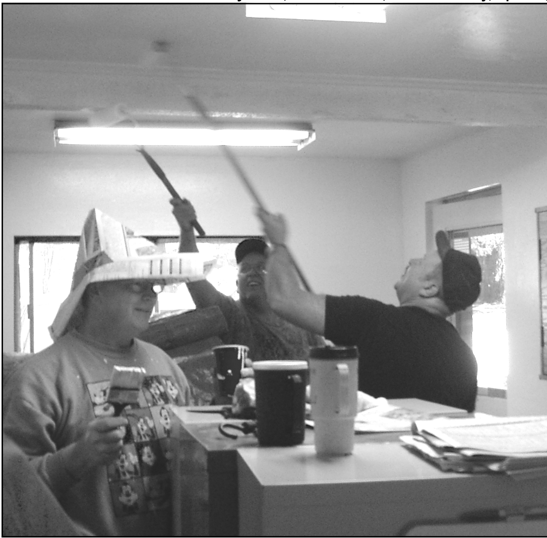
STATION PAINT PARTY - Several Illinois Valley Fire District volunteers joined Chief Harry Rich; and Beth Beards, district administrative assistant, for a work party in the main station in Cave Junction on Saturday, April 24. The goal, which was reached, was to improve the office décor, as it needed a facelift. Although a new station is planned, it was decided to make the main office more attractive for customers and staff. And Rich (wearing nifty hat) found yet another use for 'Illinois Valley News.'
