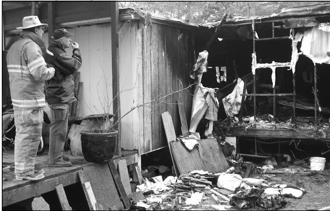
ROCKYDALE MOBILE FIRE - Illinois Valley Fire District (IVFD) Fire Marshal Jerry Schaeffer and IVFD Capt., Steve Corwin investigate fire damage to a double-wide mobile home belonging to Tim Stetz at 6455 Rockydale Road on Thursday, Jan. 22. The fire on Wednesday evening caused an estimated $70,000 damage, and a house cat perished in the flames. Investigation was inconclusive, but electrical problems are being attributed to the fire, according to Schaeffer. (Photo by Michelle Binker)
