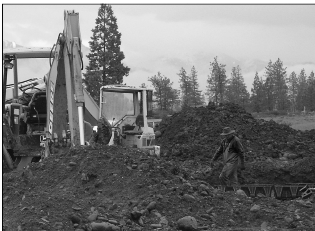
AIRPORT BUILDING GROUNDWORK - Work is continuing on a business incubator project under Illinois Valley Community Response Team. Funding consists of $500,000 from the USDA's Rural Utility Service and approximately $200,000 from Josephine County. The project is to provide a central location for new or existing businesses to utilize common services. Current work is being handled by TJ Bossard Consulting Engineers, Copeland Sand & Gravel, and Ed's Backhoe.
