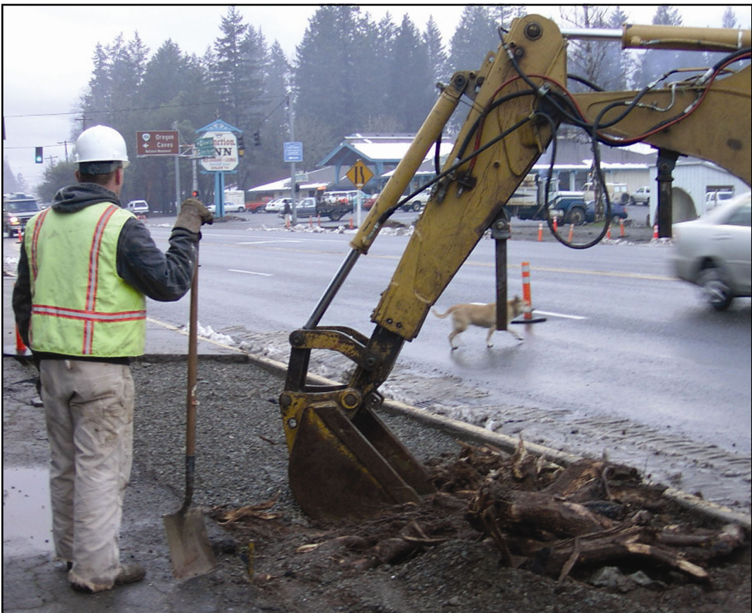
Work is progressing on sidewalk renovation in CJ. (Photo by Shane Welsh)
