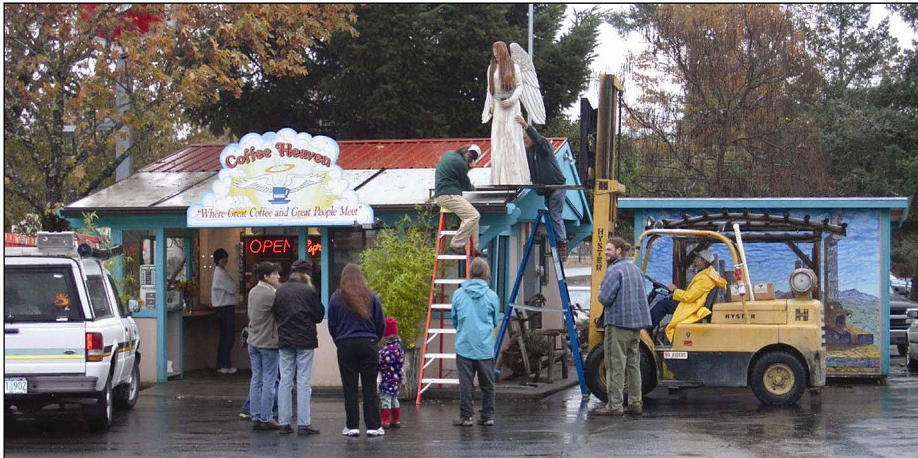
ANGEL ARRIVES - Coffee Heaven received a new angel carving on Thursday, Nov. 6. A number of area residents stopped by to watch as the large angel was lifted and placed on the top of the building. This is the second angel to grace the roof of the building. The other carving was stolen in February. The new angel has a revised look including a different face, different wings and hair. (Photo by Steve Fairchild)
