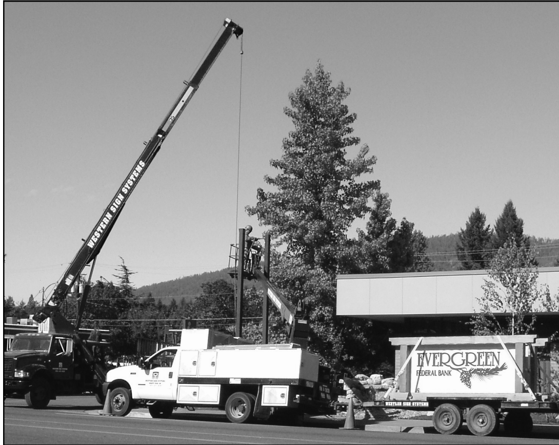
SIGN OF THE TIMES - Everyone can be on time now that the new Evergreen Federal Bank's time and temperature sign has been installed in Downtown Cave Junction. The sign is part of improvements being made inside and out at the bank.
