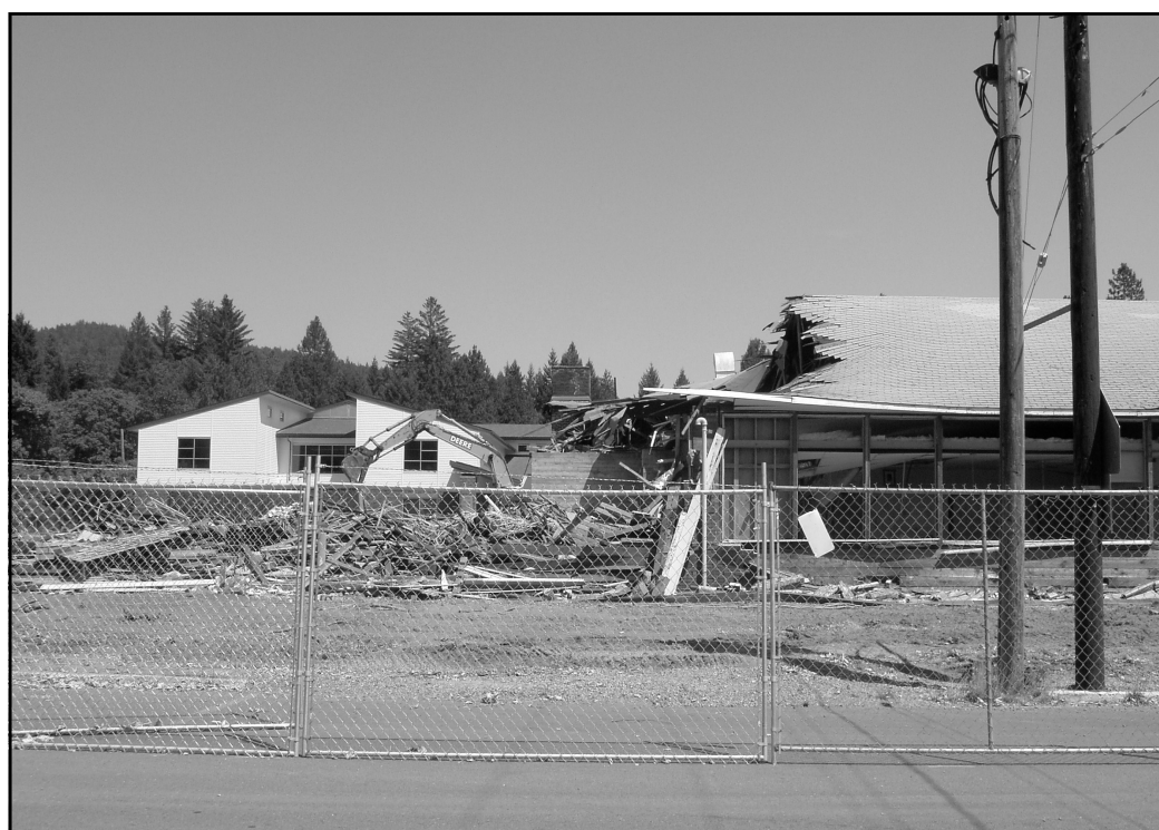
OLD AND NEW - The old Lorna Byrne Middle School is partially torn down revealing some of the new middle school building. Crews started removing the old school Tuesday, July 22.
