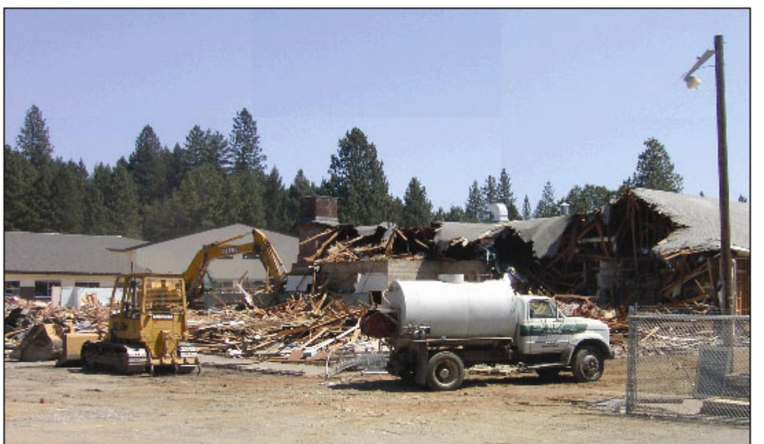
HEAVY-DUTY DEMOLITION - Workers began tearing down the north portion of the main building of Lorna Byrne Middle School, the original I.V. High School, on Tuesday, July 22. The new school complex that has been constructed, is set to open for classes in the fall, and will be visible from South Junction Avenue.
