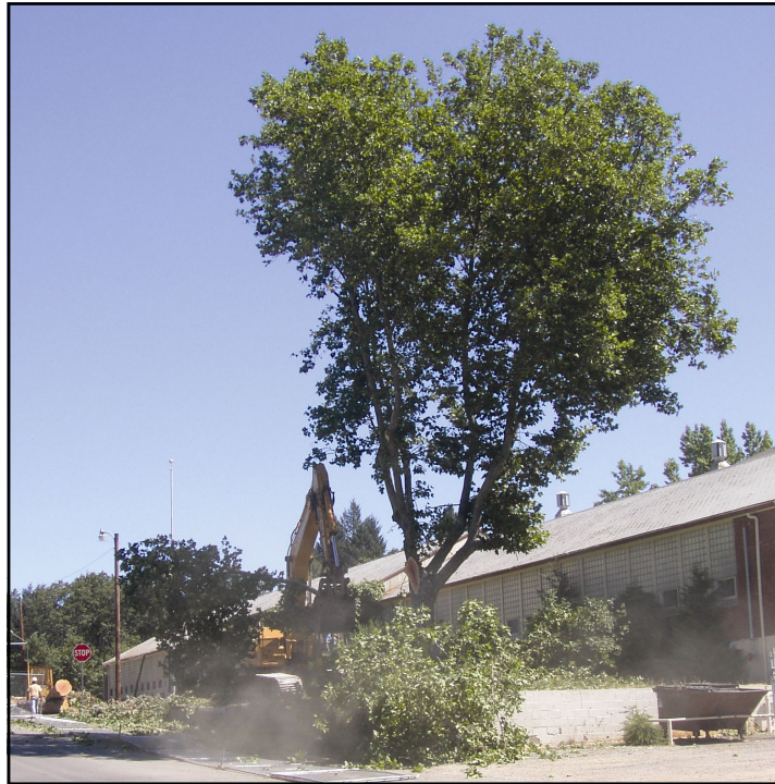
LAST GIANT - The final tree in front of Lorna Byrne Middle School fell on Monday, July 14. The six trees that lined North Junction Ave. were removed as part of the construction of the new school's parking lot. Demolition of the former wood shop building has begun at the north end of the school.
