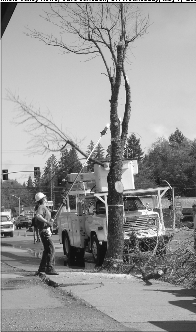
TREE REMOVAL - A number of trees are being removed from Downtown Cave Junction under a $1,600 contract by city of CJ with Marty's Tree Service. Trees being removed are damaging sidewalks and will be replaced later. Metal grates will surround new trees, and sidewalks repaired. The city began planning the project two years ago with public meetings.
