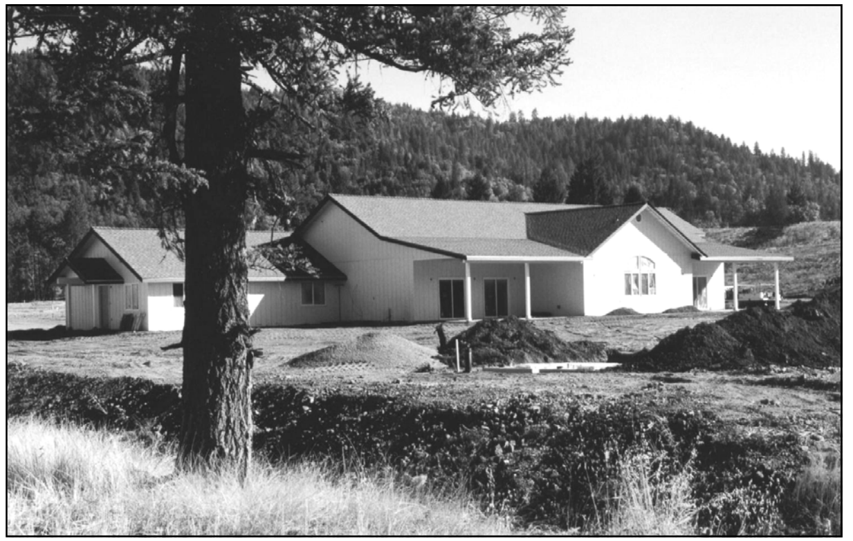
SUNNY BROOK CLUBHOUSE -- Work on the clubhouse at the new Sunny Brook Mobile Home Park on Laurel Road is nearing completion. The first phase of the development, by John Constanzo of Aptos, Calif., will include 44 sites. Streets and water/sewer lines are installed; and landscaping is under way. Mobile home models are to be available in approximately three weeks. The 25-acre site is to be developed in three phases with a total of 120 to 125 sites.
